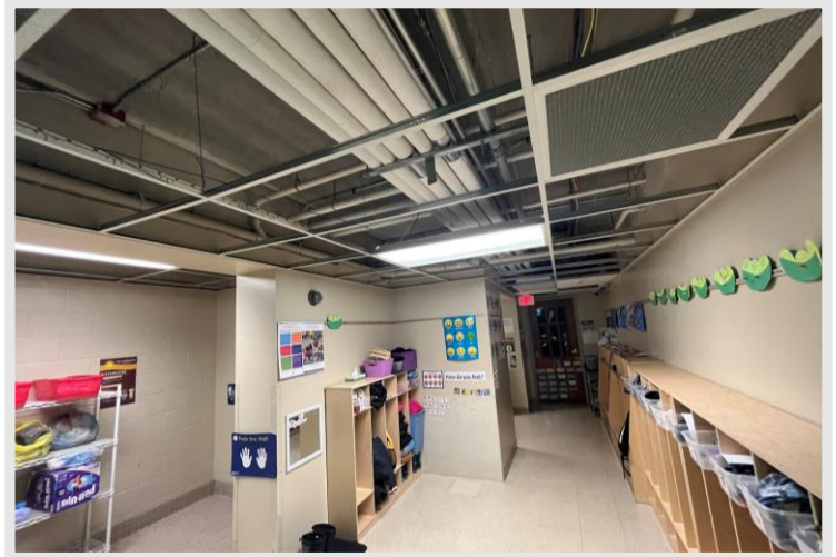
Ceiling tiles are being selectively removed throughout the building to allow for new “MEPF” systems to be planned and coordinated
