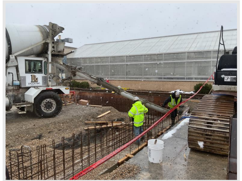
Findorff crews working through “spring” weather to pour concrete stoop footings in place and prep for foundation wall pours.
