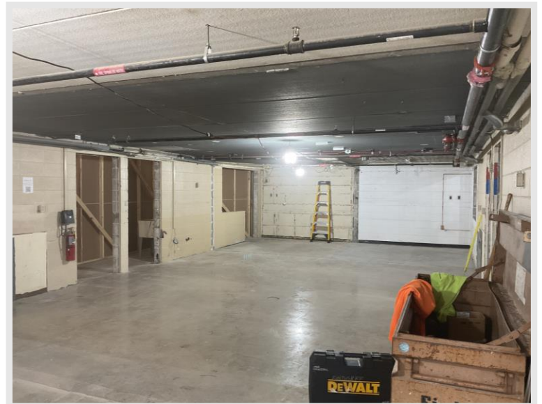
Findorff crews working on demolition of the existing rooms beneath the Maintenance/Woods mezzanine to open up for new spaces.
